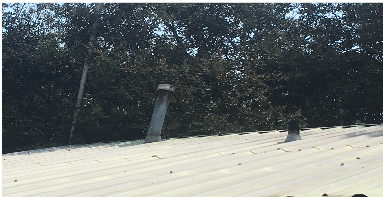
Photo 2: Close-up of Assumed Asbestos Roof Mastic on vent and pipe penetrations.
